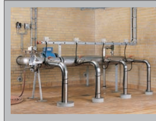
Multiple pumps can draw from an underground cavern
