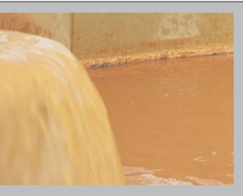
Particles in the raw water can cause pump wear
