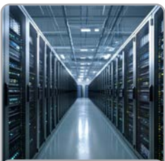
Data Center Cooling
